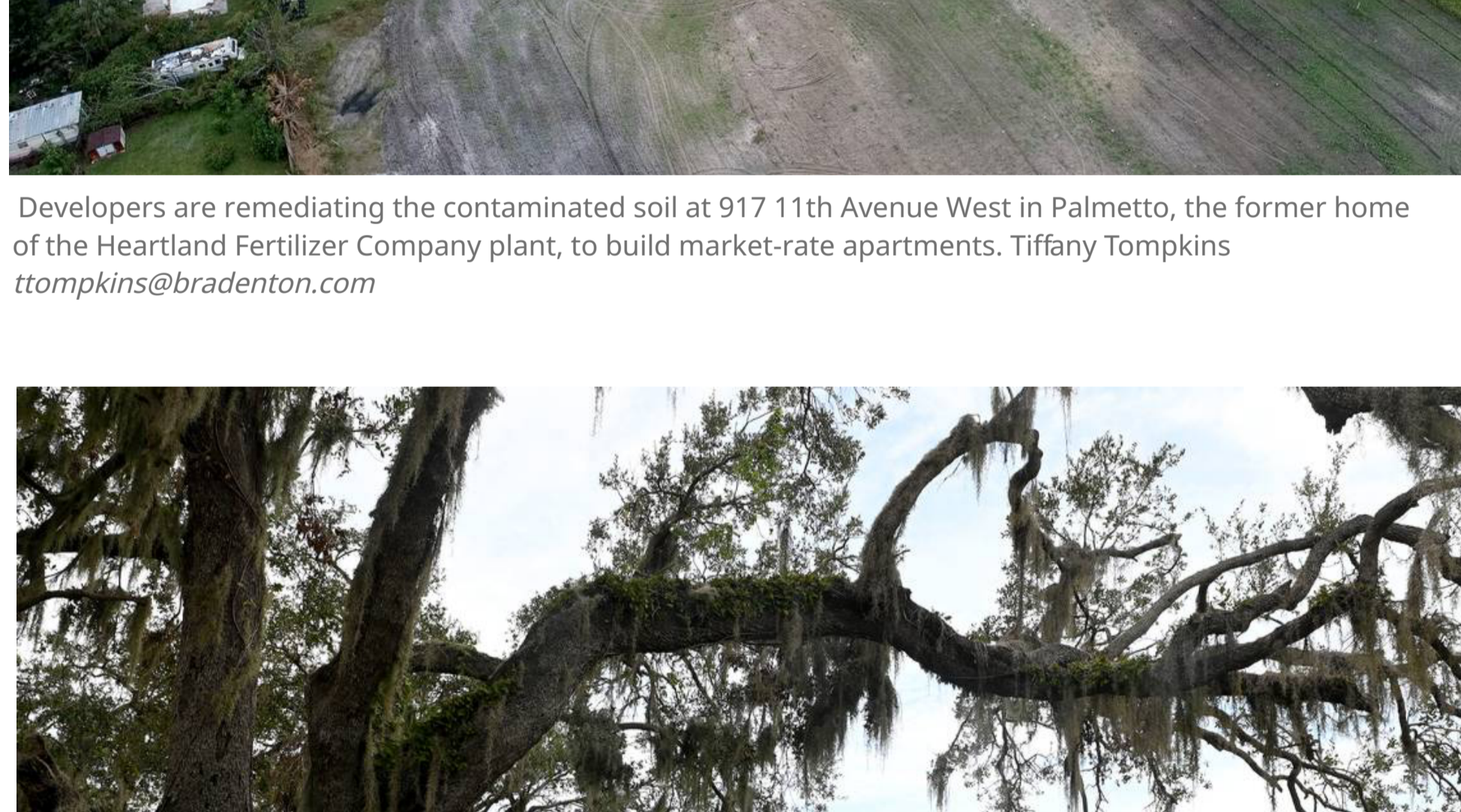
Developers are remediating the contaminated soil at 917 11th Avenue West in Palmetto, the former home of the Heartland Fertilizer Company plant, to build market-rate apartments. Tiffany Tompkins ttompkins@bradenton.com
